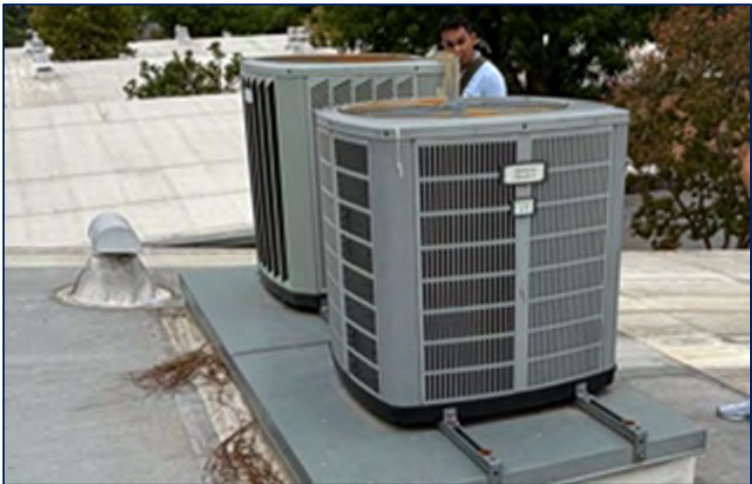
Rooftop condenser unit at Administration Building
