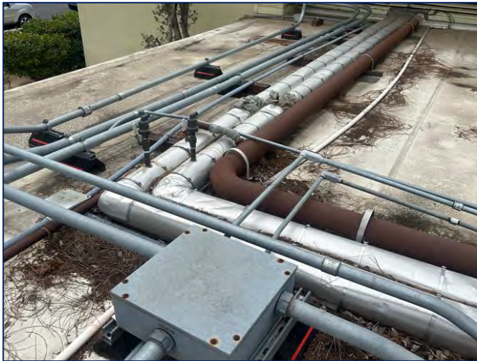
Rooftop central hot water loop
