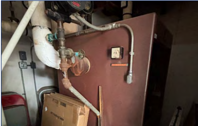
Classroom Building A boiler unit
