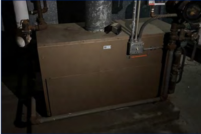
Multipurpose Building boiler in mezzanine
