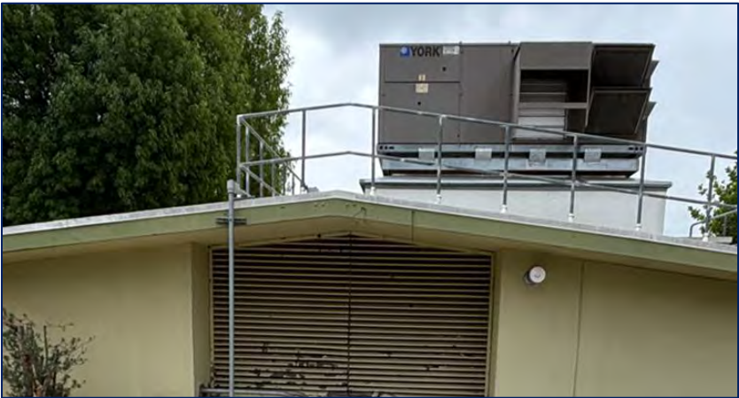
Rooftop package unit at Assembly Building
