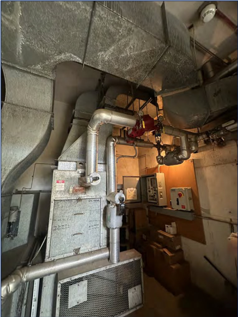
Multi-zone heating fan unit at Library Building
