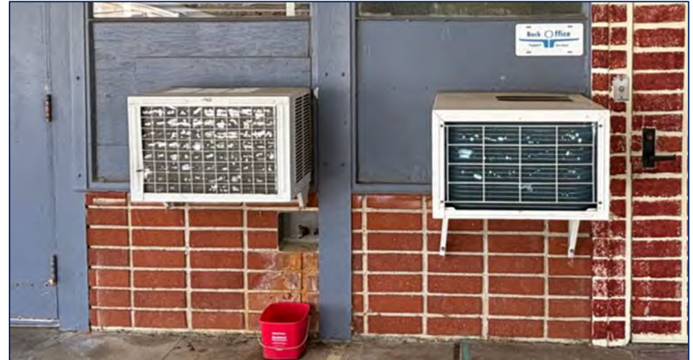
Administration Building package wall unit
