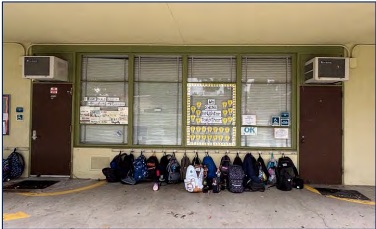
Typical classroom transom package units
