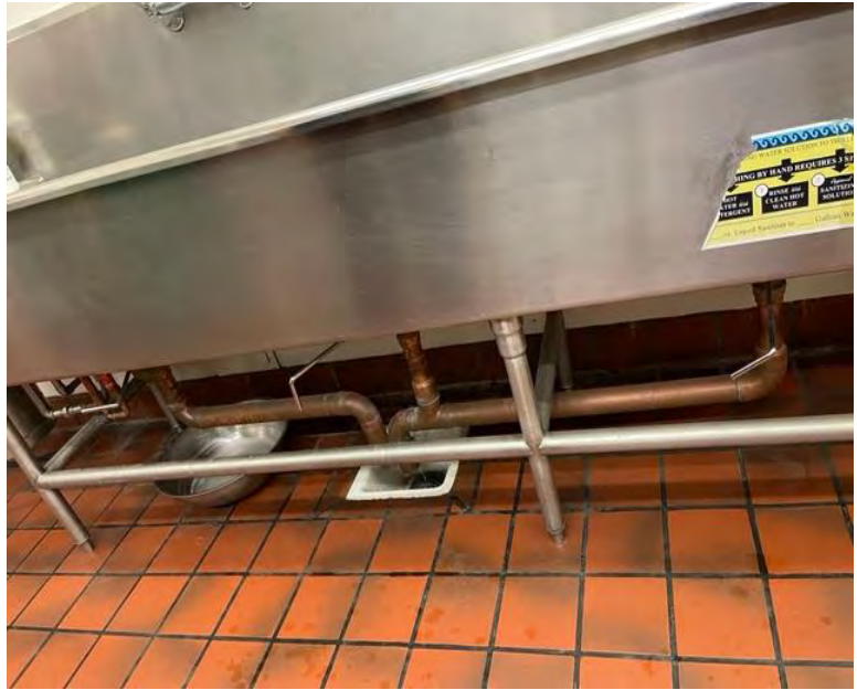
Kitchen Sink w/pipes, disposal conduits and drain fittings
