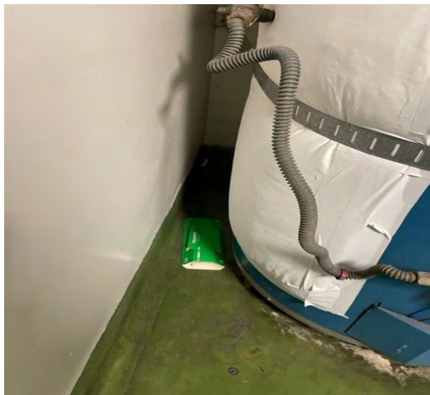
Pest Trap located behind hot water tank in the Cafeteria Kitchen @ 135 th Elementary School
