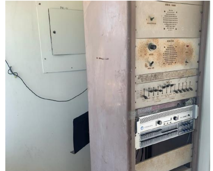
Deteriorated audio rack at athletics field
