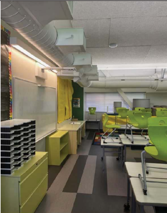
7. 2nd Floor Classroom (Inside) with Duct Silencer
