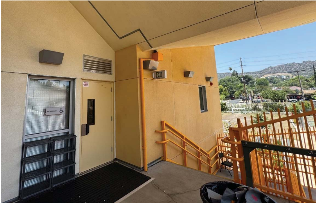
Figure 7. Dahlia Heights ES-Roof Downspout on Second Floor Classroom 2 Entry Area (OIG Photo - June 25, 2025)
