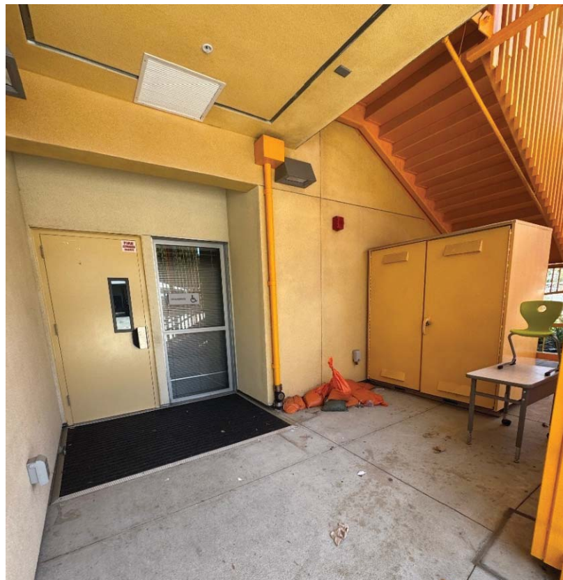
Figure 6. Dahlia Heights ES-Roof Downspout on First Floor Classroom 1 Entry Area (OIG Photo - June 25, 2025)
