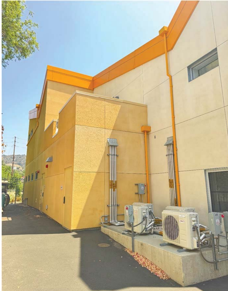
Figure 23. Dahlia Heights ES- View of Southwest Building Exterior Walls (OIG Photo - June 25, 2025)
