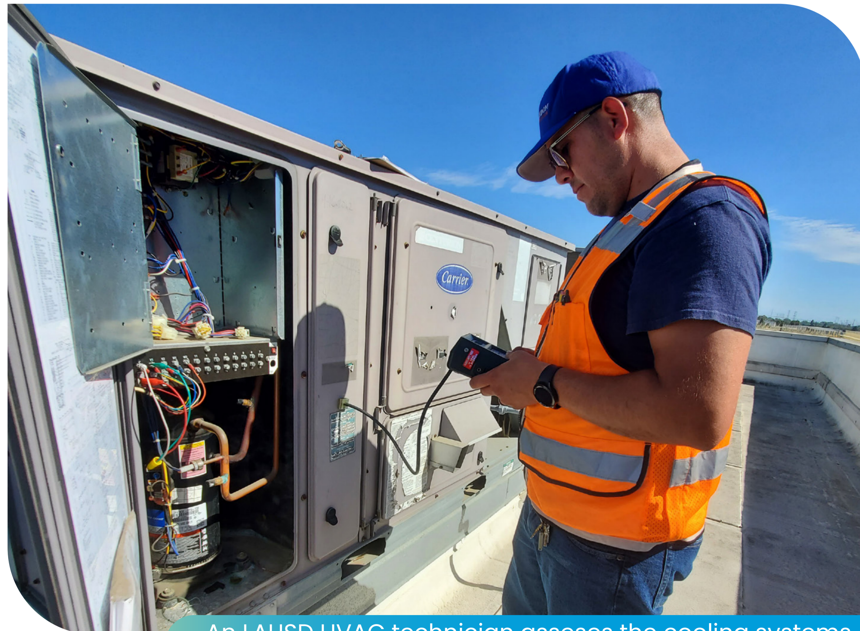
An LAUSD HVAC technician assesses the cooling systems at Rancho Dominguez Preparatory High School
