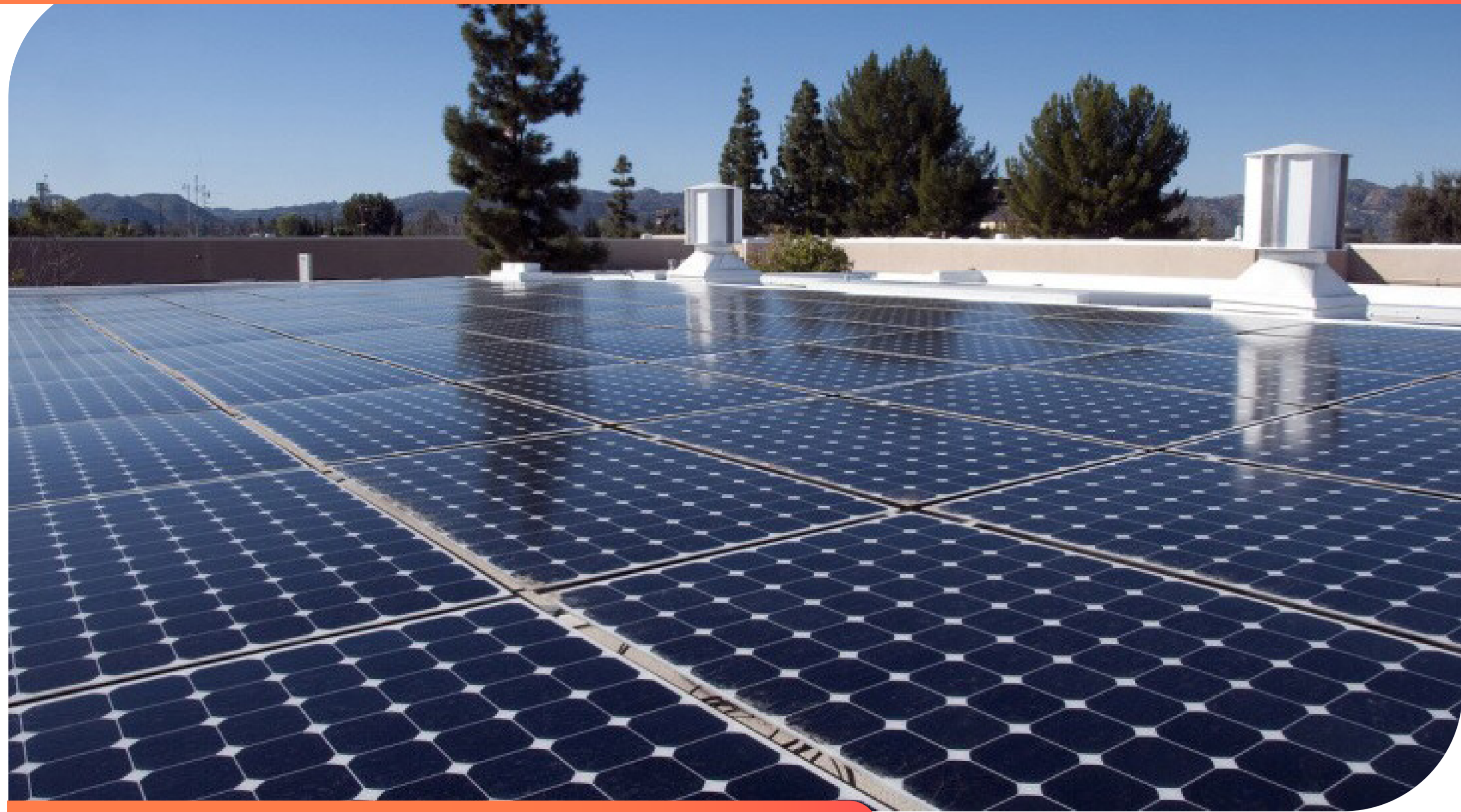
Rooftop solar array at Canoga Park High School
