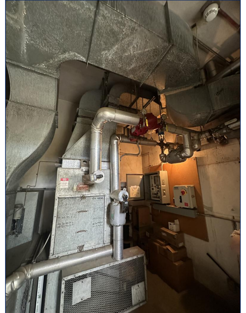
Multi-zone heating fan unit at Library Building
