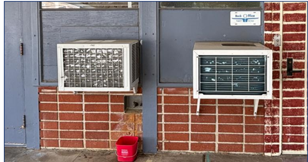
Administration Building package wall unit
