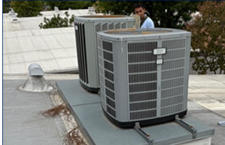
Rooftop condenser unit at Administration Building
