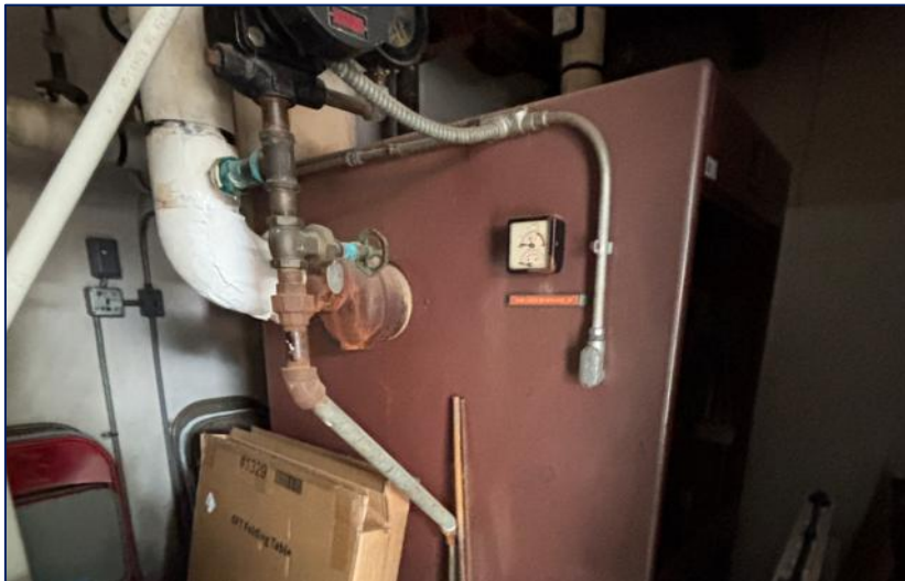
Classroom Building A boiler unit
