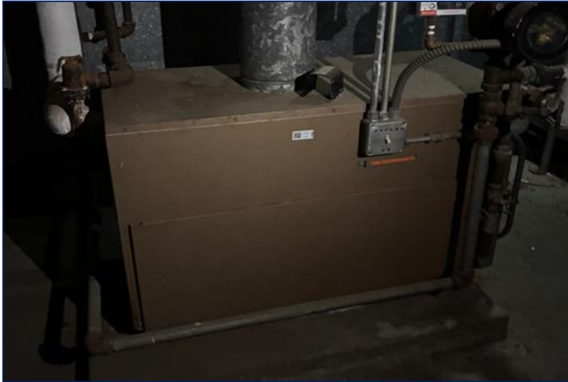
Multipurpose Building boiler in mezzanine
