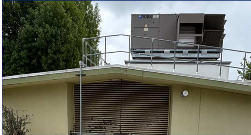
Rooftop package unit at Assembly Building
