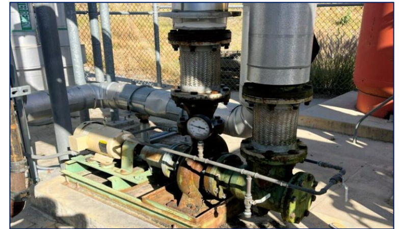
Deteriorated re-circulating pump for chiller
