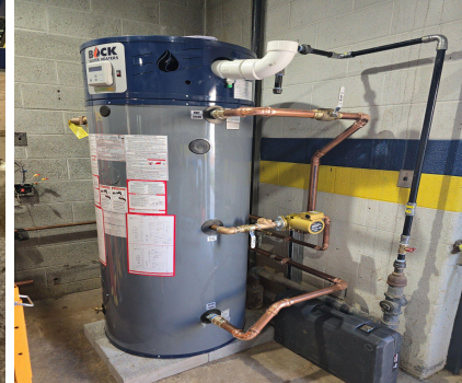
New B.6 Hot water heater
